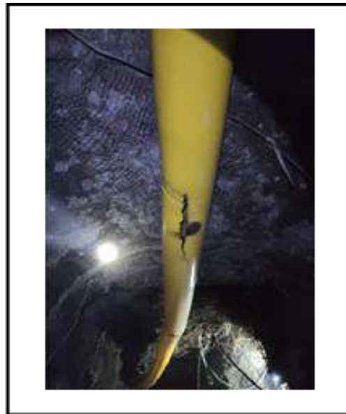
Figure 6. Holes in the flexible duct at RD KKRB 4 Utama at observation distance 2
