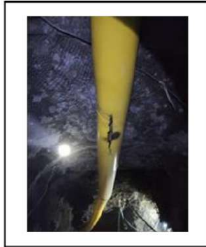
Figure 6. Holes in the flexible duct at RD KKRB 4 Utama at observation distance 2
