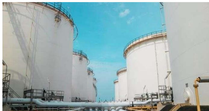
Gambar 1.3 Fasilitas Fisik Tank Storage
